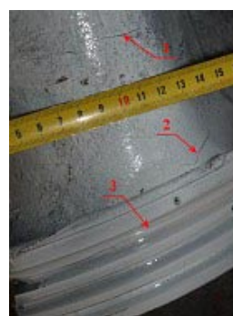
Fig. 1. Cracks identified by magnetic method in three areas
